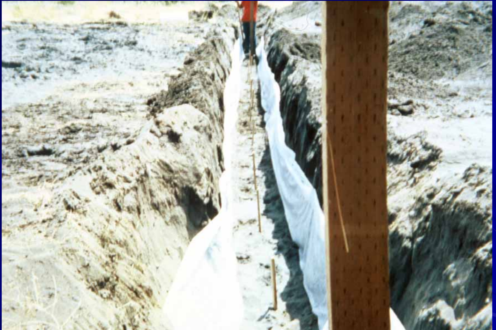
Filter fabric placed on side walls to prevent infiltration of blow sand
