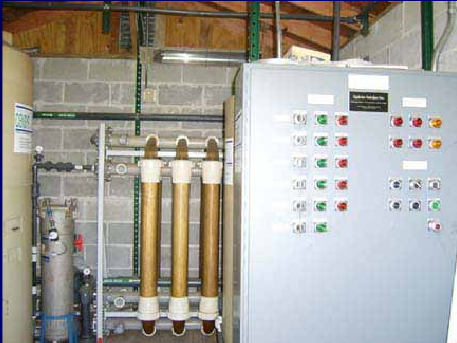
Membrane Filtration system installed to treat HSW— system did not work
