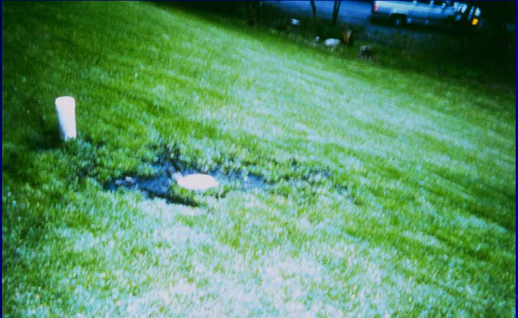
Steep slope—leaking mound
